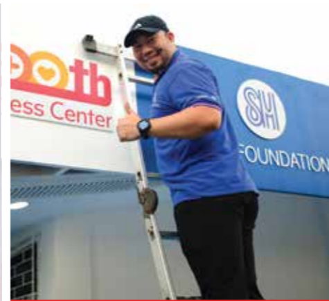
SM Foundation's Senior Project Manager Albert Uy places the 200th Wellness Center marker as they complete the final stages of the renovation.
