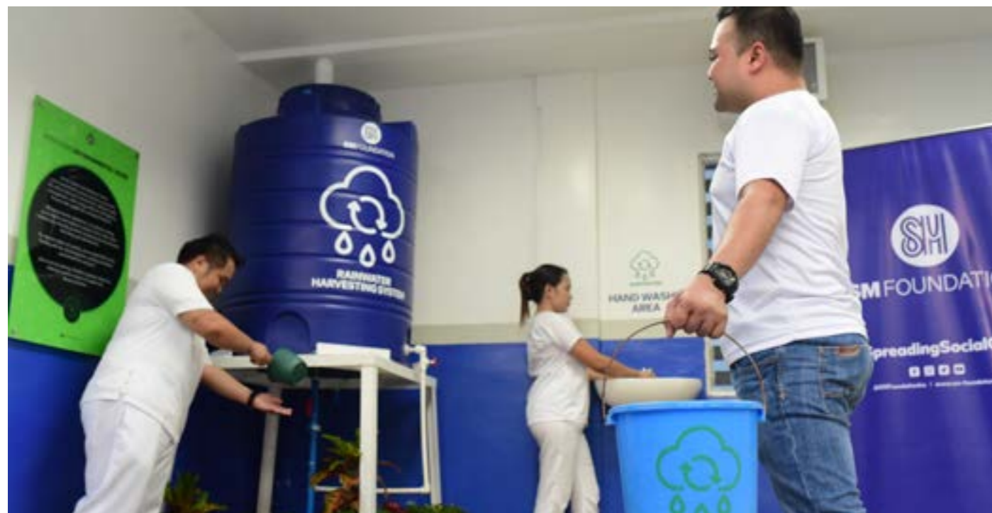
The staff of the health center conveniently access water from the Rainwater Harvesting System for various non-potable uses.
