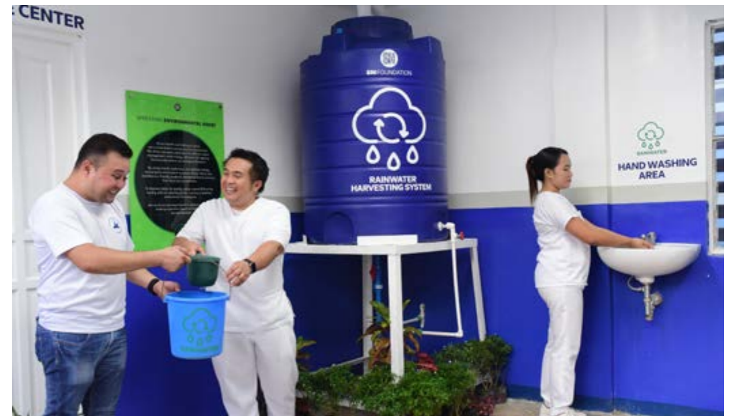
Promoting water conservation, SM Foundation installed a rainwater harvesting system in San Fernando, Cebu Primary Care Facility
