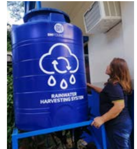
Midwife Narcisa Jagmis observes as the system collects rainwater from the gutters.
